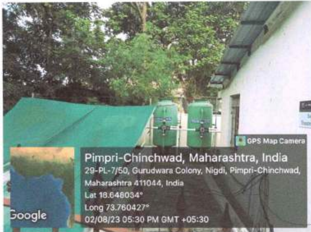
Geotagged photograph of Sewage treatment plant at D Y Patil Educational Complex.
