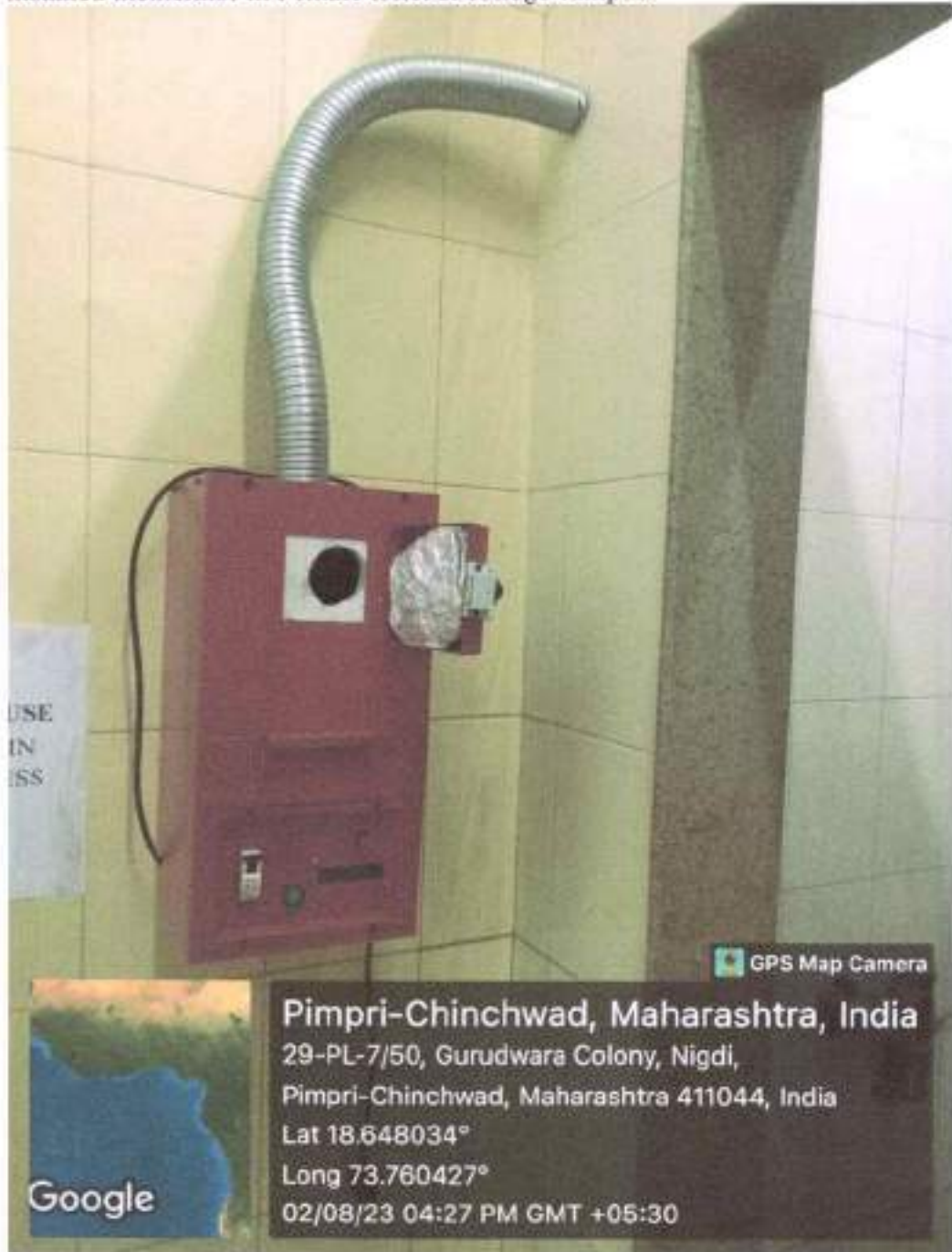
Geotagged photograph of incinerator at female toilet of college campus.
