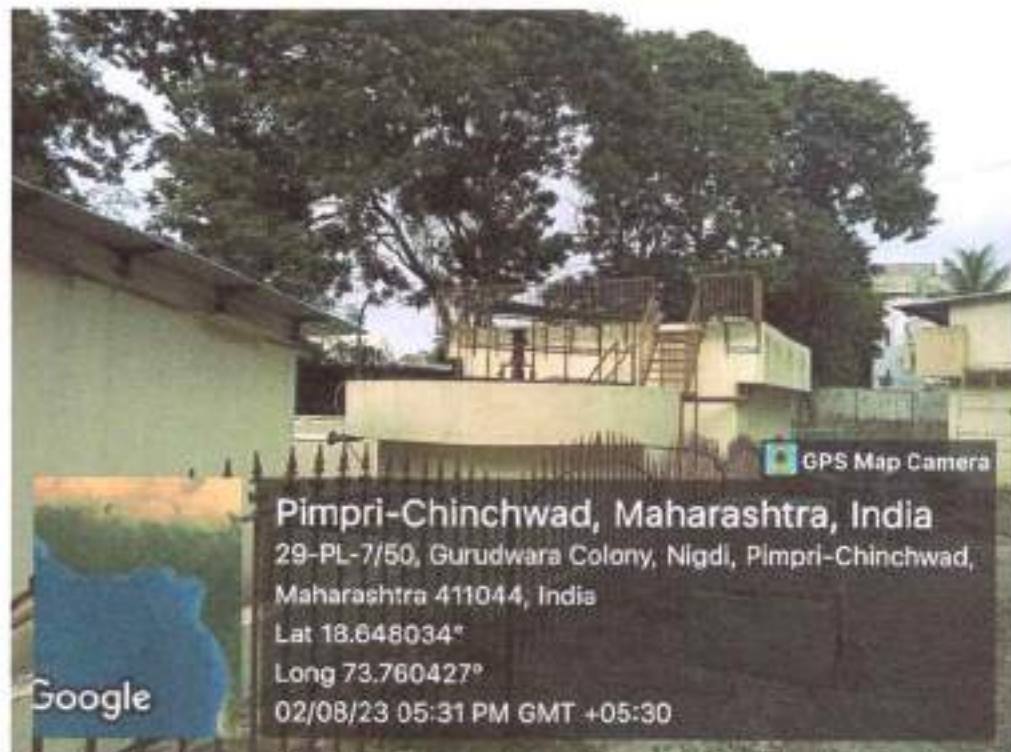
Geotagged photograph of Aeration tank in STP at D Y Patil Educational Complex.
