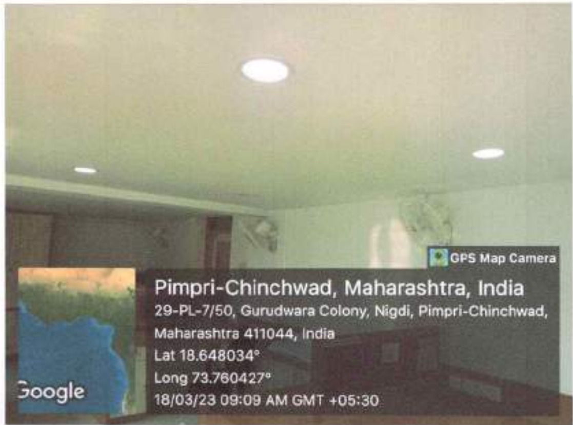
LED installation in the staff room. Each ceiling Luminaire have 20W and wall fan have 60W.
