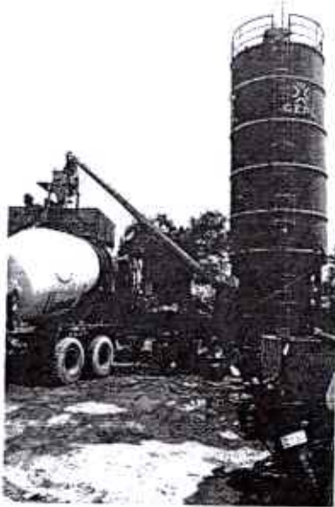
RMC Plant, Urban Skyline Ravet, Pune
