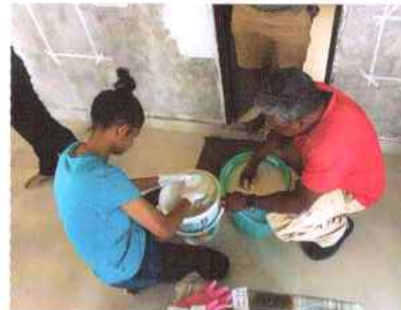
3. MIXING OF LIME PLASTER ( BEFORE APPLICATION POWDERED LIME SOAKED IN WATER OVERNIGHT )
