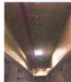
65 DIA CPVC PIPES RUNNING IN THE Lobbies
