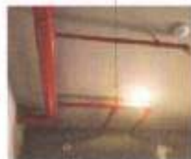
SMOKE COLLECTOR HOOKED FROM THE SPRINKLER HEAD
