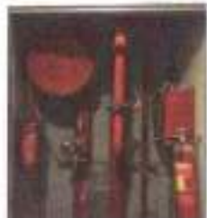
FIRE FIGHTING EQUIPMENT IN THE SHAFT
