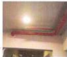
80 MM DIA CPVC PIPES COMING FROM THE MAIN VERTICAL SHAFT
