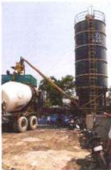
RMC Plant, Urban Skyline Ravet, Pune
