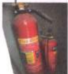
FIRE EXTINGUISHERS OF CLASS A AND CLASS C
