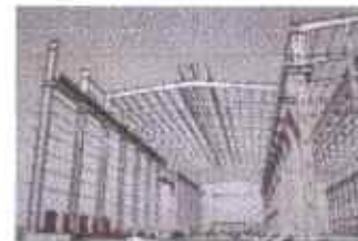
Fig. no. 10: Column and beam erection. Source: MGS (Modern green structures) Architecture (Online)
