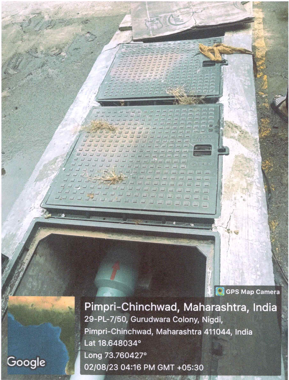
Geotagged picture of rain water harvesting chamber to borewell.
