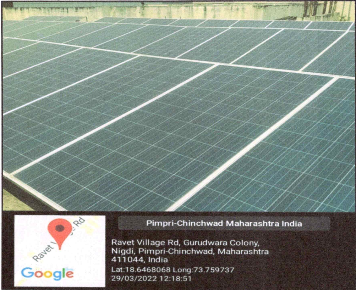
Geotagged Photograph of On grid Solar PV Plant at D Y Patil Educational Complex
